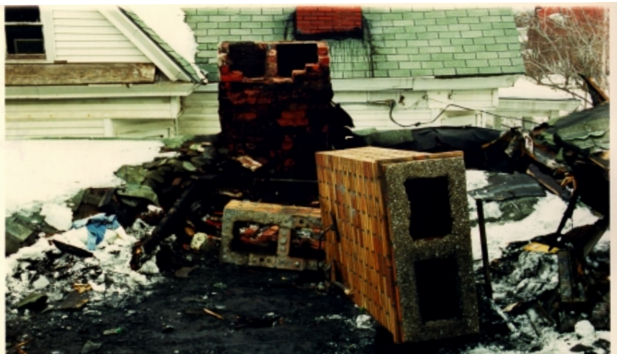
Figure 2. Collapsed brick chimney
